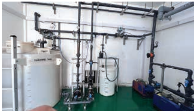
Sewage treatment plant at Pullman Maldives Maamutaa Resort
