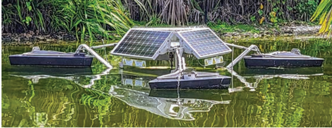
SolarBee water purifier at Pullman Maldives Maamutaa Resort's natural lake
